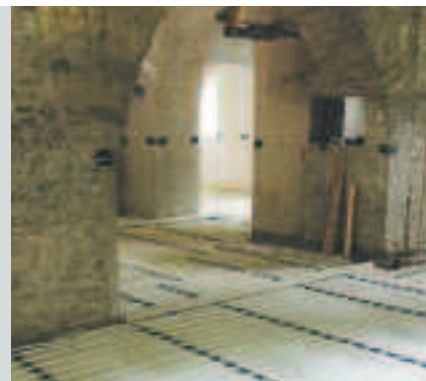
St Teilo's church: Under-floor pipework being laid inside the church on top of a limecrete base. The flagstone floor acts as a heat reservoir and the system is controlled by hydrostrats located in the roof-space.
