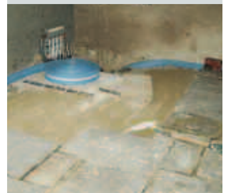
St Fagans Castle. Electric under-floor heating was introduced into the kitchen, the flagstone floor acting as a heat reservoir.
